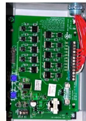
Reverse Jet Pulse Timer Assembly Mounted In NEMA 4 Enclosure & Prewired to Solenoid Valves
